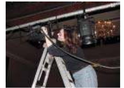
In addition to performing on stage, Kristin Danko '05 lends a hand with the wiring.
